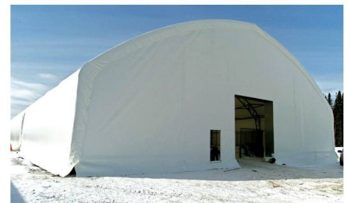
Work is underway in covering this UFS Phoenix structure for an ice hockey facility in Alberta, Canada.
